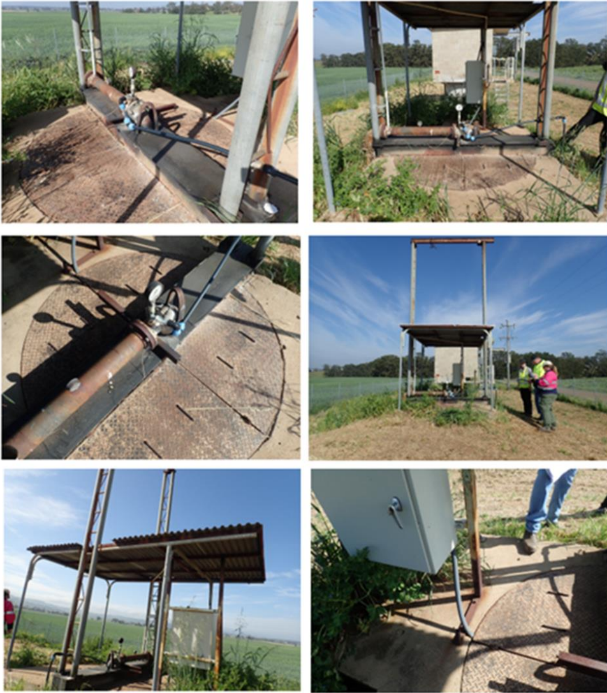
Figure 7 - Coolah Back -up Well
